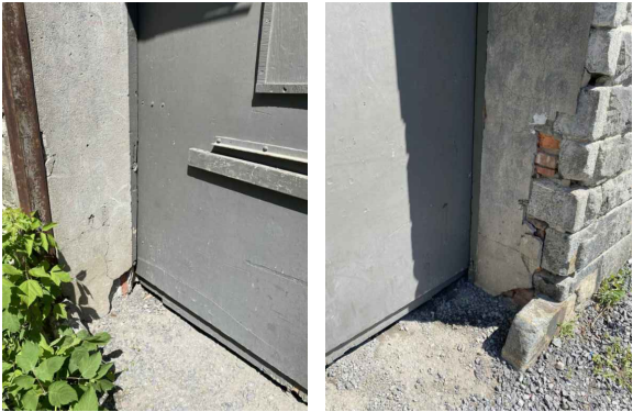
PHOTOS 1.1 AGRANDI ANCRAGES
